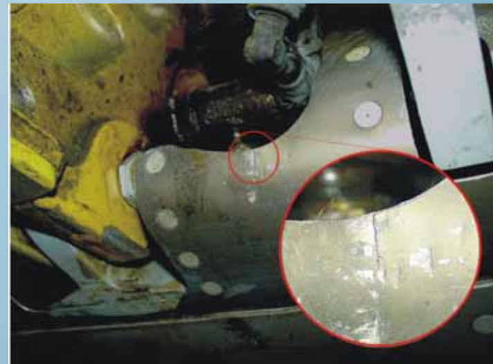
Visual Crack Indication
